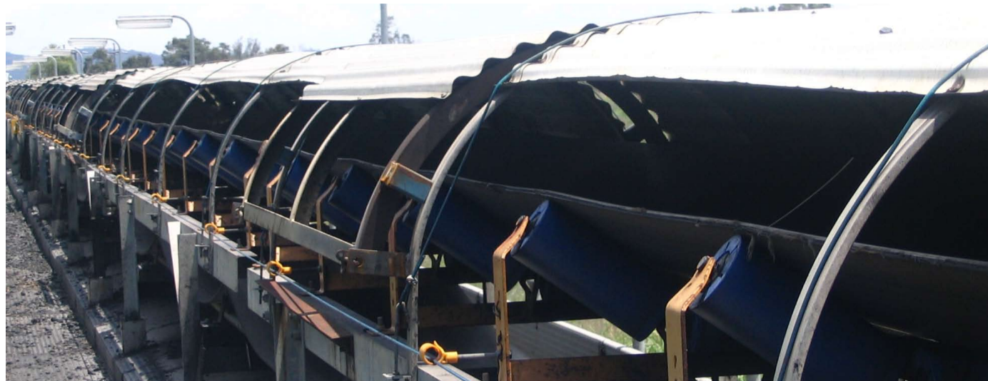
Steel rollers on the surface conveyor are progressively being replaced with poly rollers (blue).
