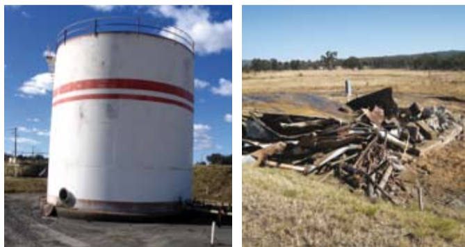
800 kilolitre bulk diesel tank before and after.
